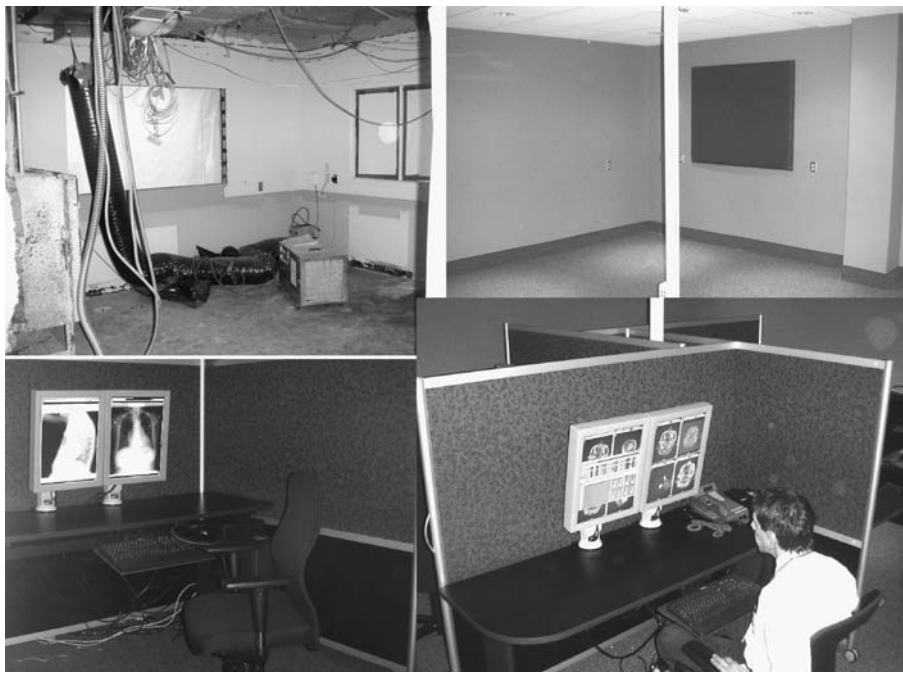
FIGURE 13.12 Different stages of the conversion of a clinical space into a reading room for radiologists. Note the pinwheel-shape design using the center floor of the room. Power and networking are supplied through the column in the center of the floor.
