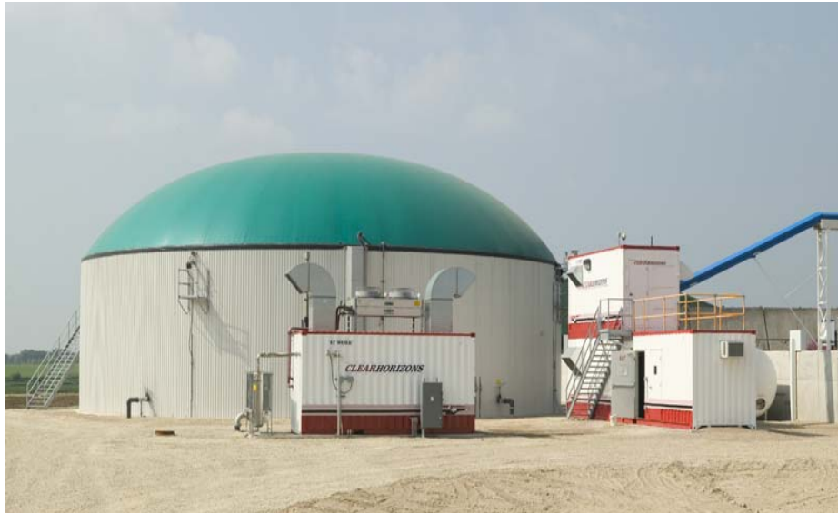
Figure (4.1): Rubber top digesters [23]
