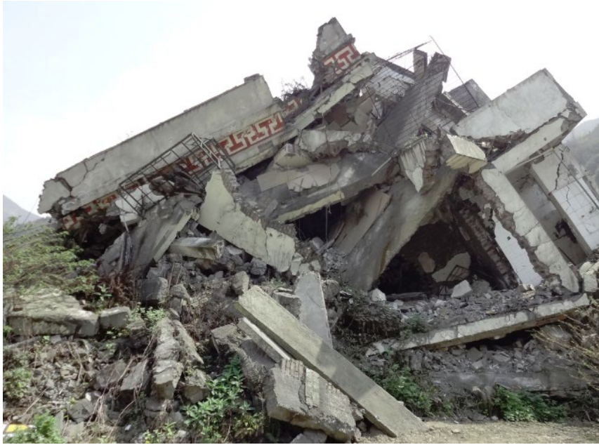
Figure 5.1 Damaged building by the Great Sichuan Earthquake, China, 2008
