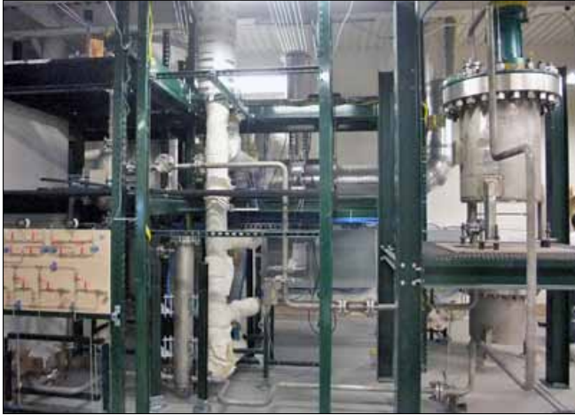
Fluoride test facility (Sun)
